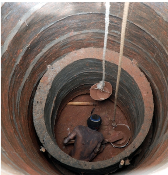
The freshly cleaned well being sunk an additional meter to ensure good supply during the dry season. Nothing is fast!
